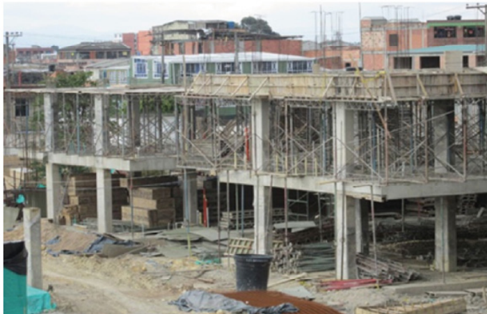
Figura 2. Unfinished works. Alianza Quiroga School in Suba.[18]
